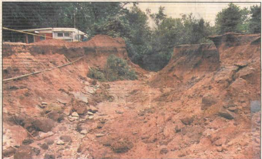
A trench dug through the city streets in Bath to direct floodwaters away from town and into the Illinois River is no longer being used.
