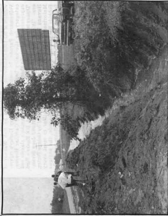
Sunday morning a trench was dug along Route 78 near the old drive-in theatre to facilitate the movement of water to White Oak Creek and into the river.
