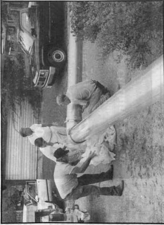
across Havana to pump water from the south end to a sewer at Jefferson and Schrader.
