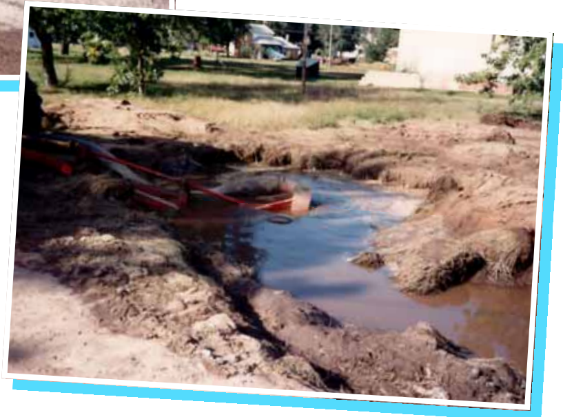
12 inch cristafoil pump in operation
