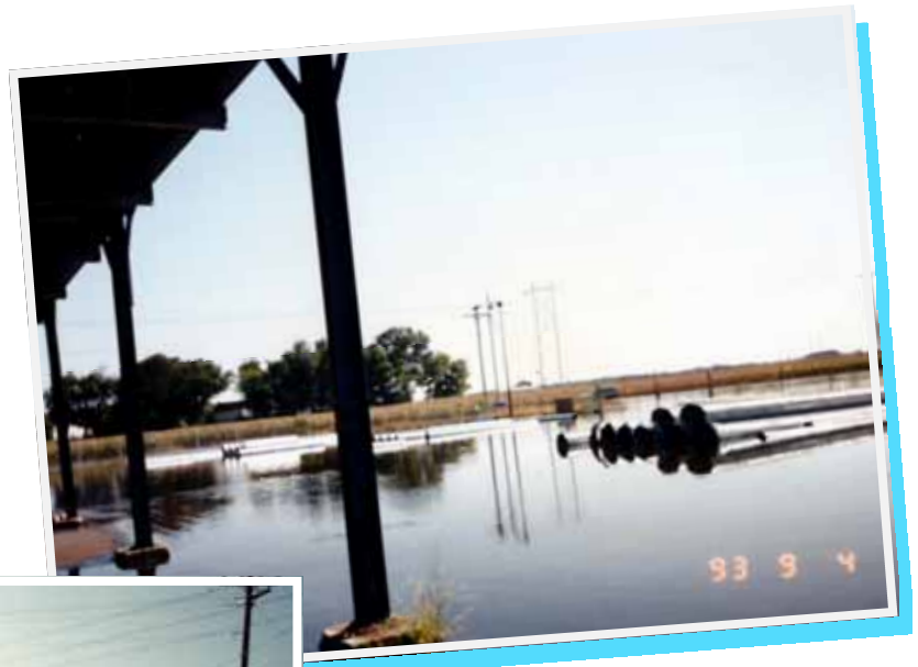
Havana Metal Culverts along IL Rte. 97 south of the railroad tracks (southeast of Havana)
